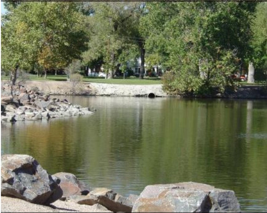
Retention ponds maintain a pool of water throughout the year and hold stormwater runoff following storms.
